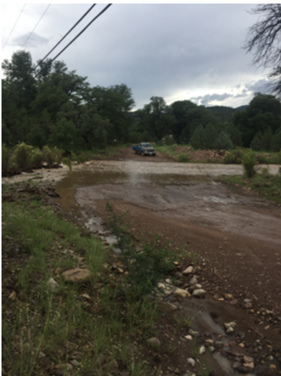
Below Fig. 1: Flash flood of a seasonal creek after heavy rains makes entrance road impassable.
